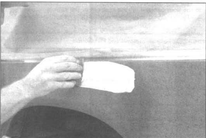
11 The primer will help reveal imperfections or scratches. Fill these with glazing compound. Follow the label instructions and sand it with 360 or 400-grit sandpaper until it's smooth. Repeat the glazing, sanding and respraying until the primer reveals a perfectly smooth surface
