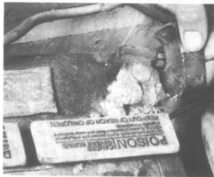
38.5A Battery terminal corrosion usually appears as a white fluffy powder
